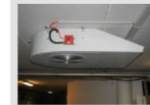
Car park fans
