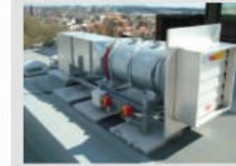
Mechanical ventilators & HVAC
