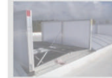
Natural flap ventilators
