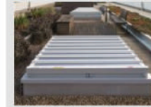
Natural louvred ventilators
